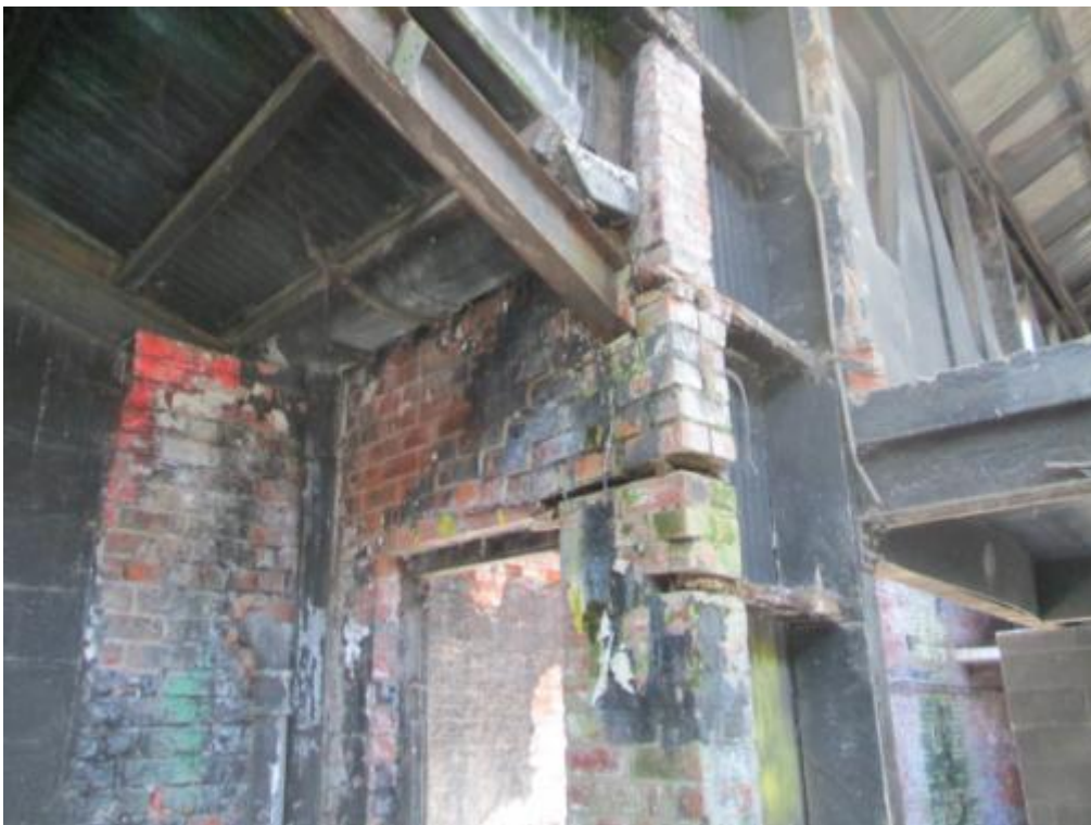
Photograph 66 – Rafter supported on wall above failed timber lintel
