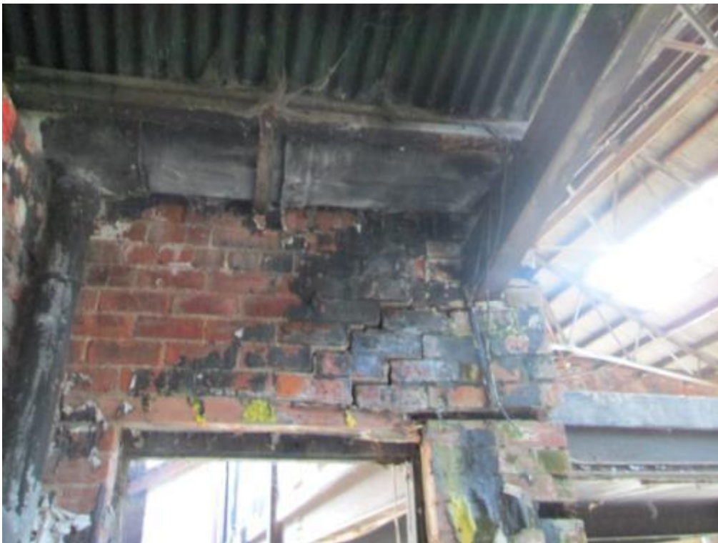
Photograph 65 – Failed timber lintel with steel rafter supported on wall
