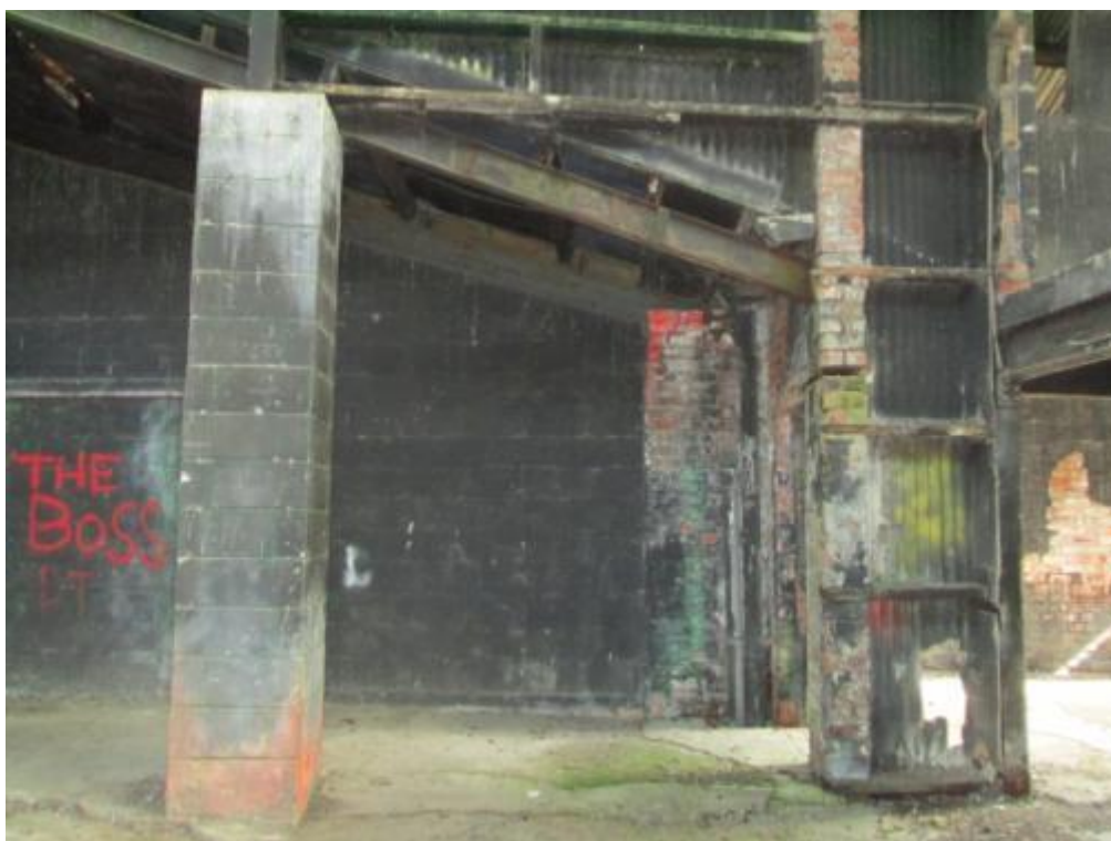
Photograph 66a – Rafter supported on wall above failed timber lintel
